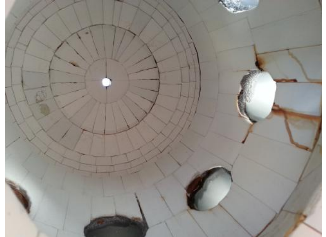
Previous distributor had a poor lining method used by a competitor
