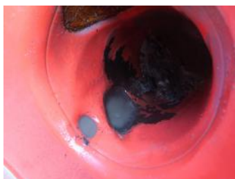
Original Rubber Lining around Outlets after 700 hours
