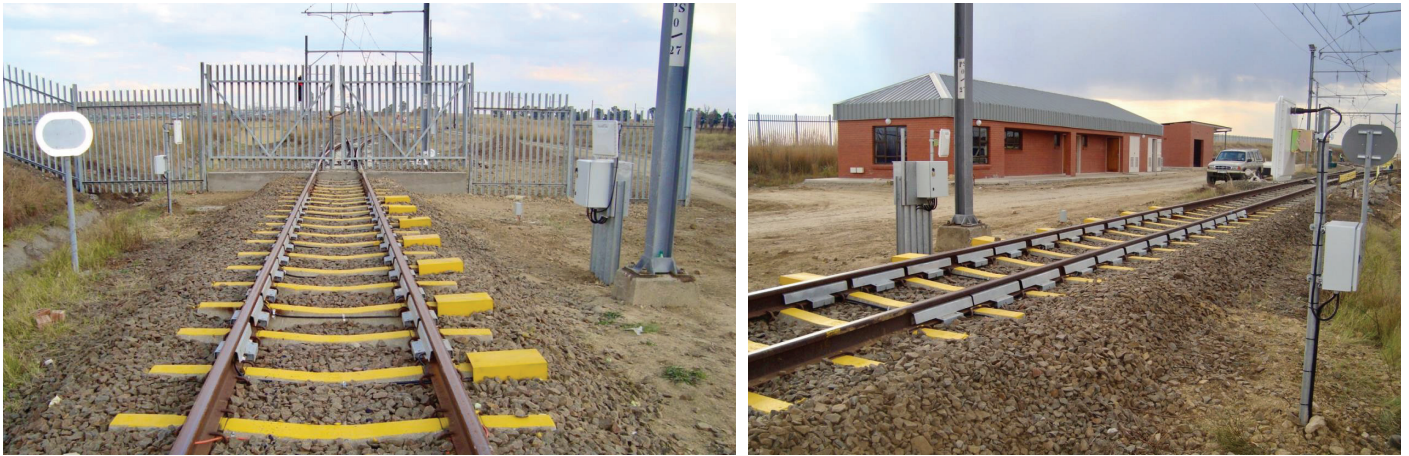
Two views of the Dyna-WIM S System, including AVI
