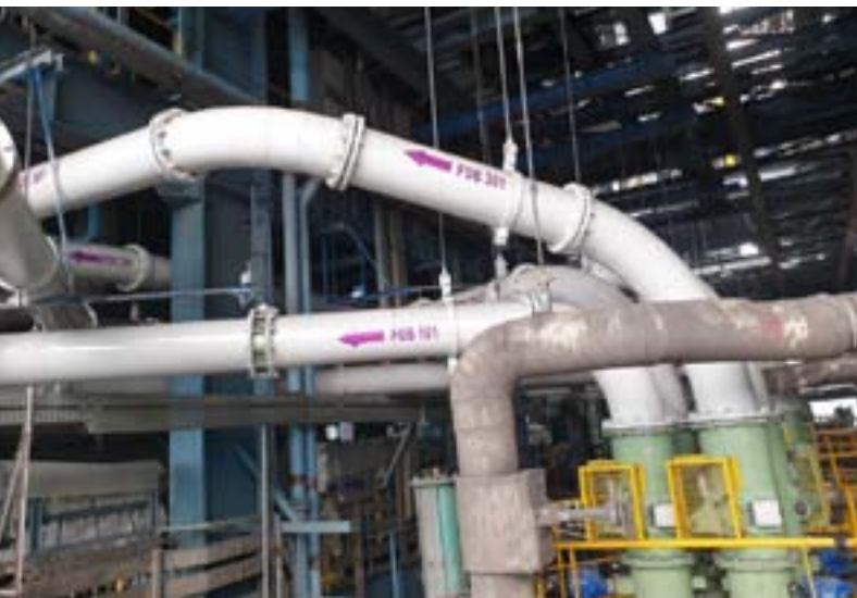
New pipework with PFMS sensor between the flanges (white) and mill isolating valves with CoalFlo® underneath (green with yellow cages around limit switches)
