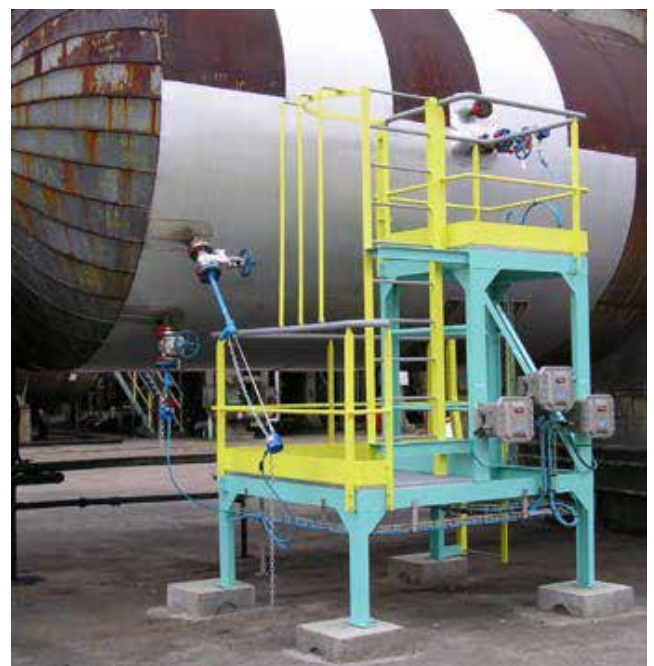
Agar ID System 2 Installation
