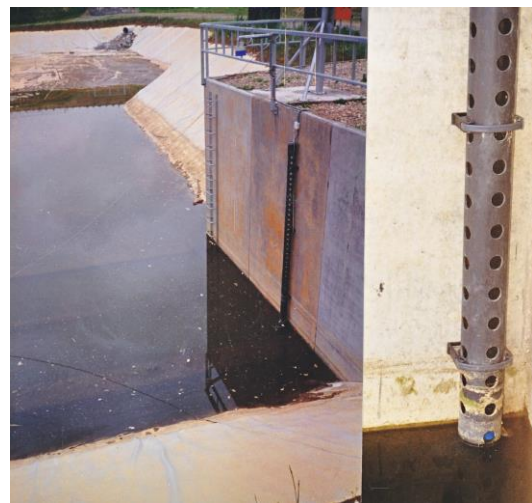
ID-221 Monitoring Runoff from a Highway Junction
