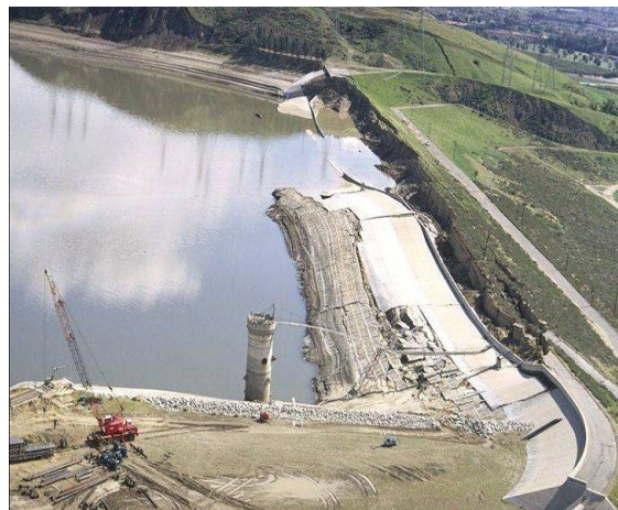
Figure 2: Photo of the San Fernando dam failure during the 1971 San Fernando earthquake
